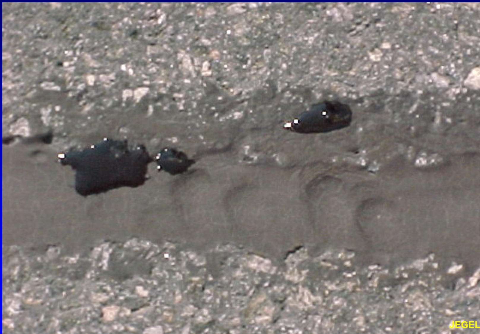
WATER TRAPPED UNDER THE CRACK SEALANT, RUNWAY 08-26, CFB GOOSE BAY
